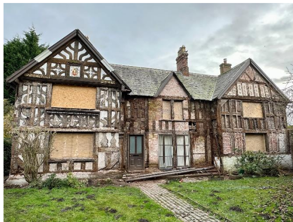
Restoration of Tarporley Manor House in progress, including improved insulation. Photo © N Gatt
